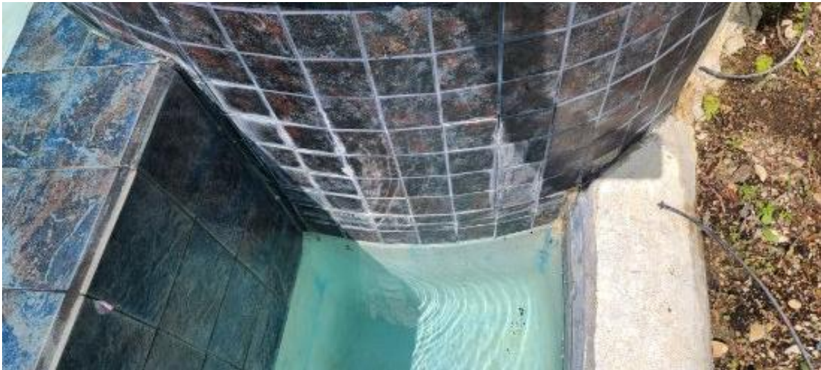
Deposits and worn grout at the tiles
