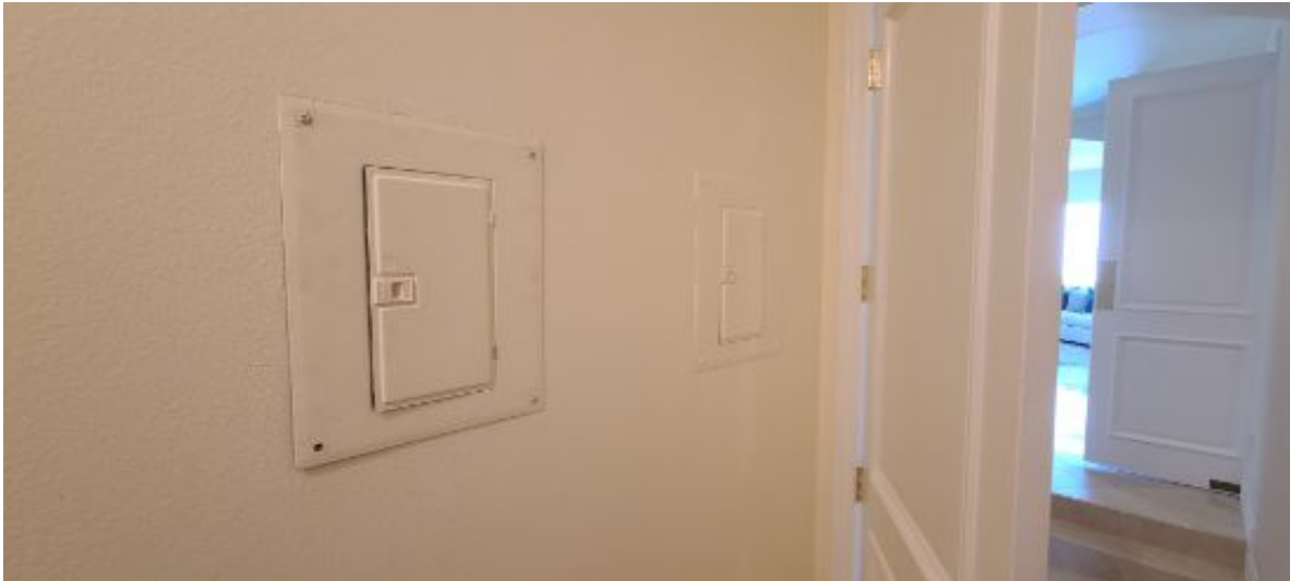
Two panels in this area
