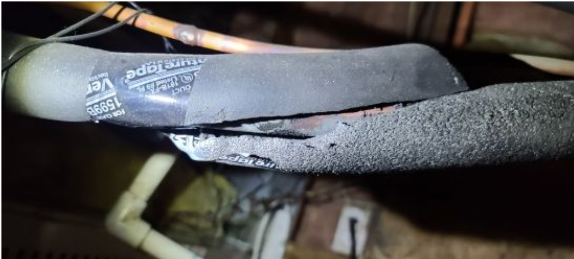
Damaged insulation needs repair.
