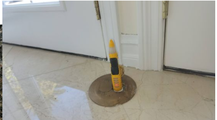
No ground in the floor outlet. This outlet is also loose.
