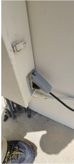
Missing weather proof covers:
