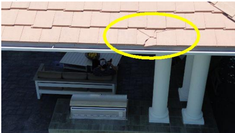
Cracked tile - over covered patio
