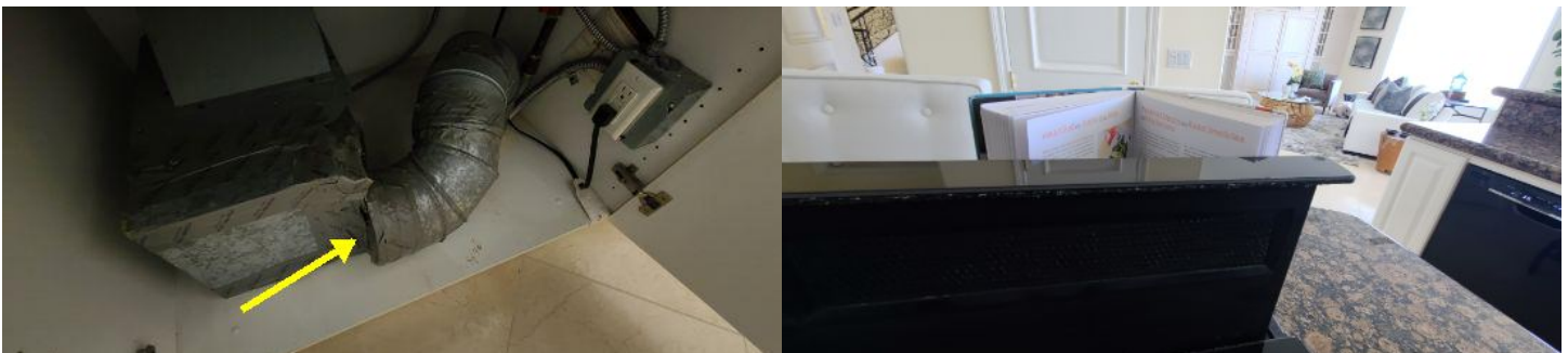
Only 1/2 of the duct is connected.
