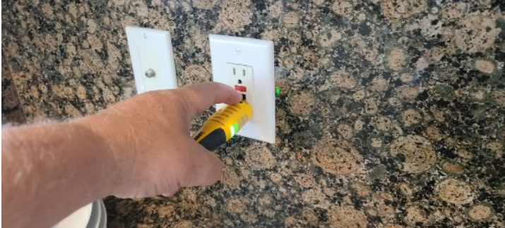
Kitchen outlets were not tripping
