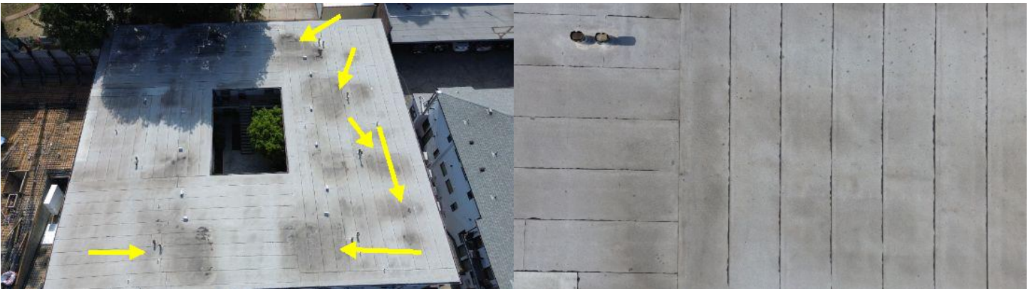
Ponding occurs in areas as the roof is very flat
