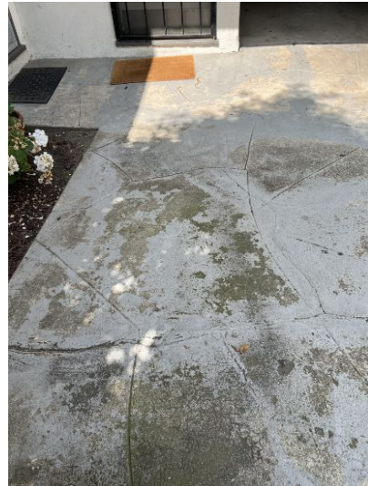
Area that may hold water due to lack of drainage.
